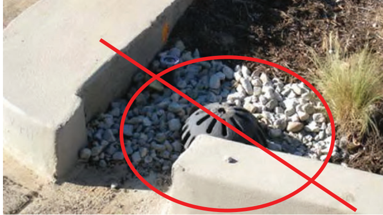
Figure 6: Incorrect Placement of an Overflow Inlet.
